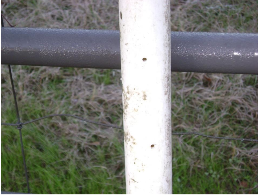
holes drill (too big) in the pipe
